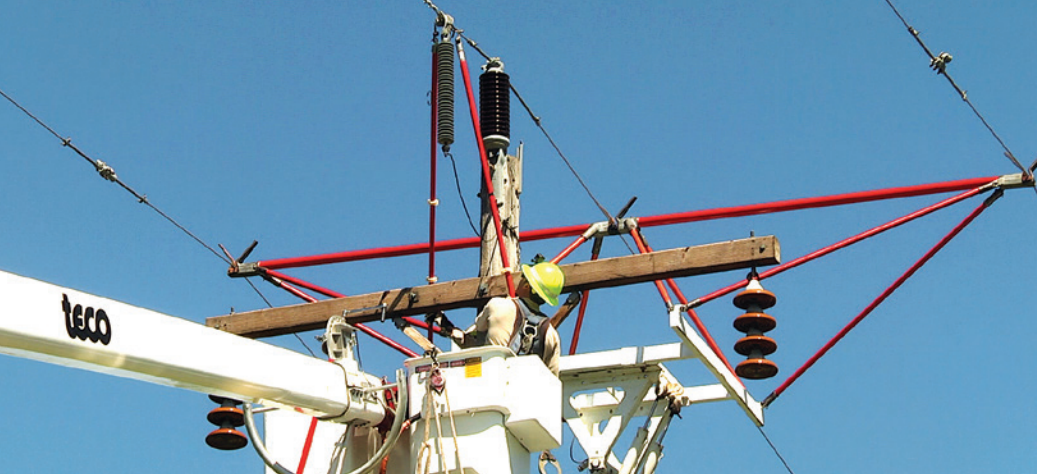
A Minnkota lineworker removes an old hanging lightning arrester on an energized 69-kilovolt (kV) line.
