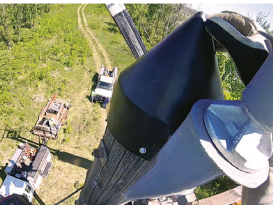
A poletop helmet is installed on top of the structure to prevent birds from nesting and perching on the structure.
