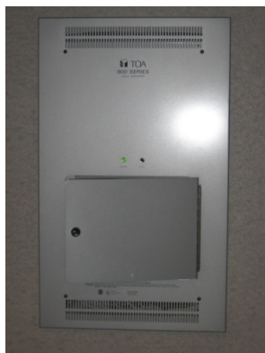
Figure 5 Sound system controls are located on the west wall
