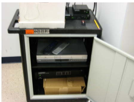
Figure 4 DVD/VCR unit is located within the cart just to the right when you enter the closet.
