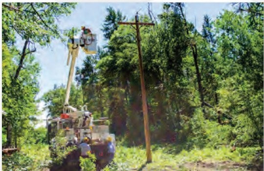
Right-of-way clearing ensures there is sufficient room for maintenance equipment and crews to access and work safely on lines.
